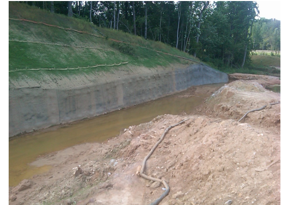
Standing water and mud after every rain
